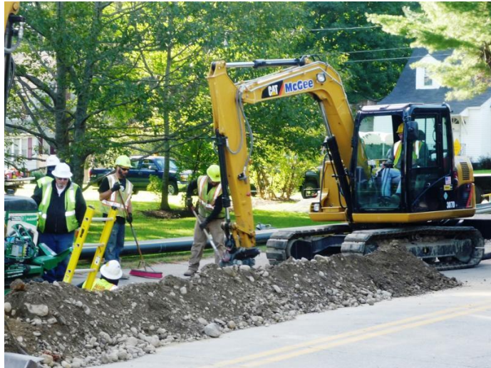
Construction crews from Summit Natural Gas of Maine install a portion of pipeline on Sewall Street in Augusta that will provide natural gas service for residents and businesses. Photo courtesy: Summit Natural Gas of Maine
